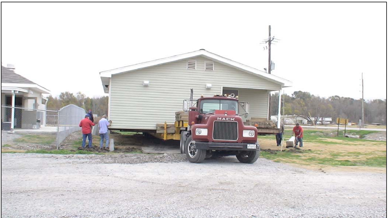
The structure is placed at the permanent site at the corner of Veterans Blvd. and Hwy 3185. Further work must be done before the facility is ready to be completely opened.
