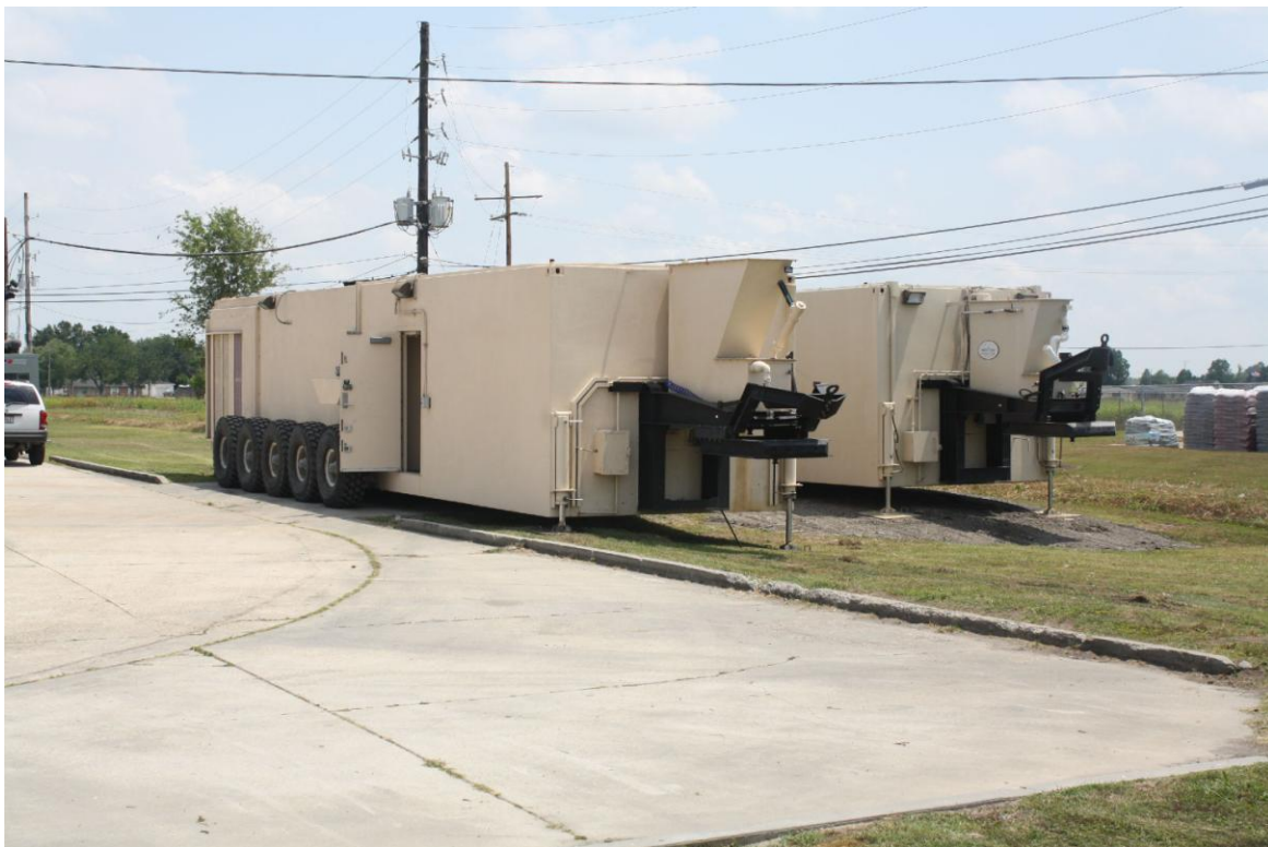
Photo of both emergency trailer units behind the Mathews Government Complex.
