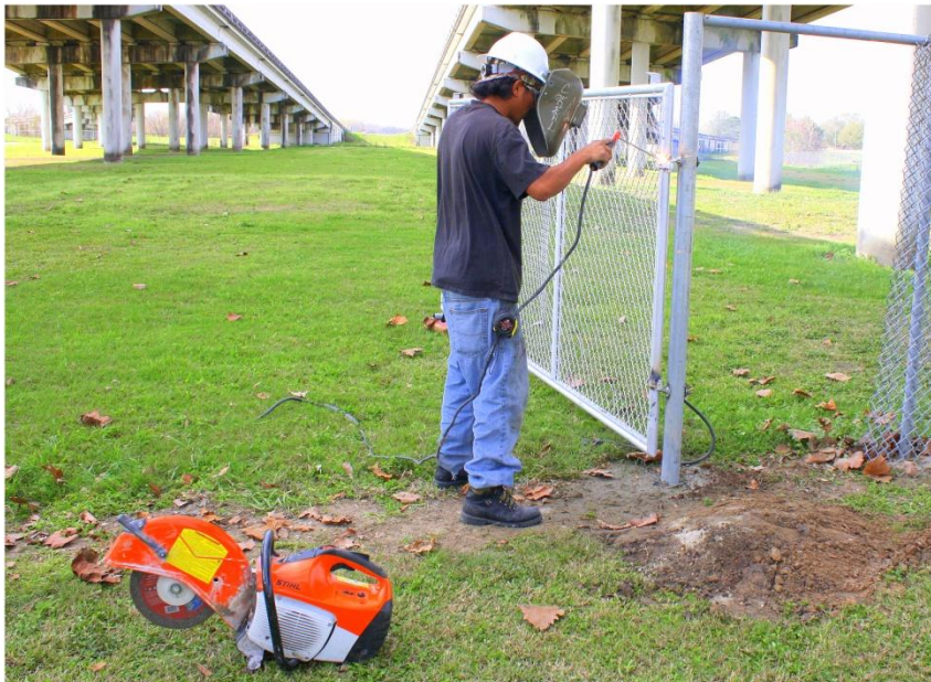
A Gulf Con crewman welds together a gate Tuesday morning at the construction site entrance of Cajun Village and Central Market under the U.S. Highway 90 overpass in Raceland.
